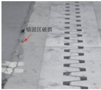
图7 梳齿型伸缩缝典型病害 Fig.7 Typical disease of cantilever-finger joints
