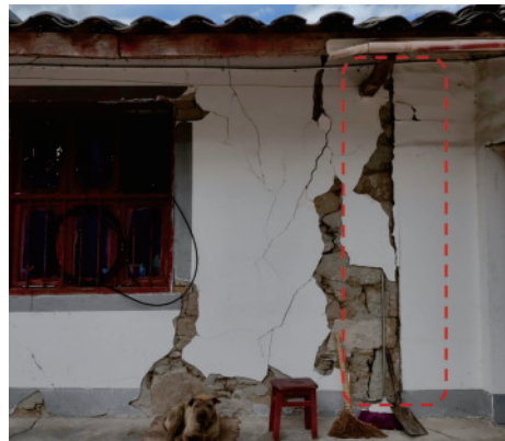
图 17 石墙开裂(德威镇,Ⅸ度) Fig.17 Crack of stone wall(Dewei town, intensity of IX)
