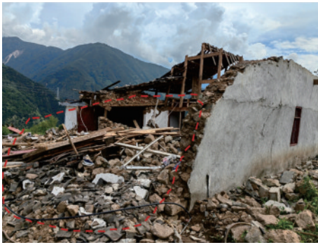
图 15 整体倒塌(德威镇,Ⅷ度) Fig.15 Overall collapse of the structure(Dewei town, intensity of Ⅷ)
