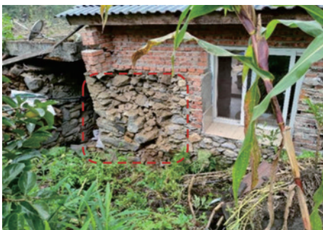
图 16 石墙剥落(磨西镇,Ⅸ度) Fig.16 Desquamation of stone wall(Moxi town, intensity of IX)
