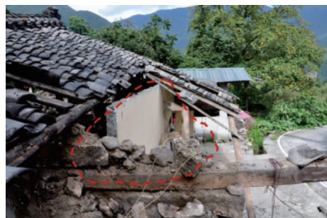
图 18 屋盖破坏(燕子沟镇,Ⅷ度) Fig.18 Damage of the roof(Yanzigou town, intensity of Ⅷ)
