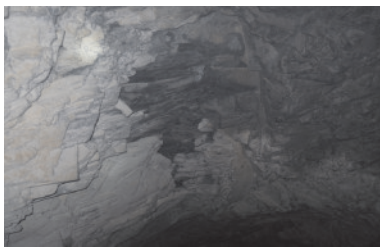
图3 内拱顶片帮现象 Fig.3 Spalling off phenomenon within the vault
