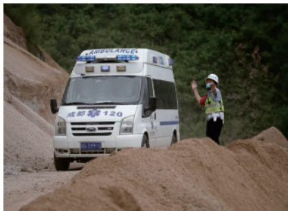
(b) S211边坡滑坡被抢通
