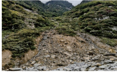
图4 坡面侵蚀 Fig.4 Slope erosion
