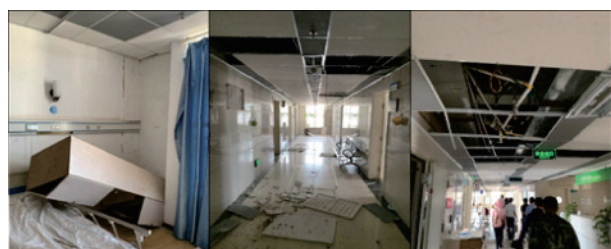
(a) 住院楼一吊顶坠落、储物柜倒损
