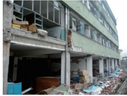
图10 梁、柱上方半高填充墙采用悬挑方式与柱顶连接 Fig.10 Masonry infills located on the cantilever beams
